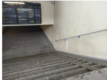
Fig. 2. Stairs and driveway in the tunnel at the main railway station in Bielsko-Biała (the authors' photography)
