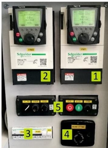
Fig. 2 Control and regulate unit: 1 – frequency converter of the driving electric motor, 2 – frequency converter of driven electric motor, 3 – box with modular breakers, 4 – central power switch, 5 – controlling regulators
