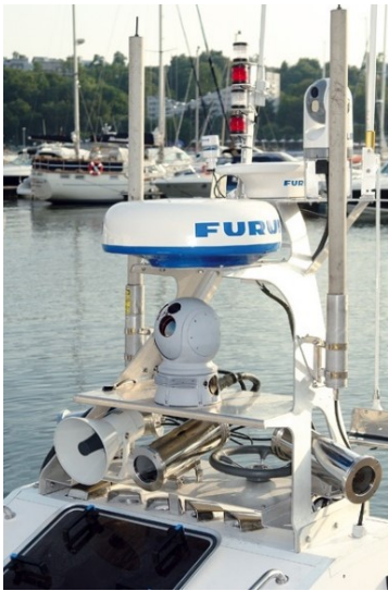
Fig. 2. The arrangement of the navigation devices and communication system antennas on the mast [R&D project No. 0 R00 0004 07 documentation]
