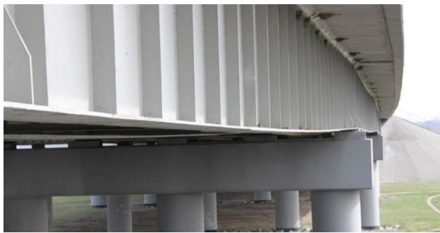
Figure 4: Permanent deflections of the girders of the main spans.
