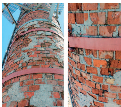
Photo 4. Technical condition of the chimney in the middle section – visible signs of surface repairs
