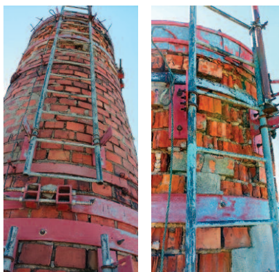
Photo 3. Technical condition of the upper part of the chimney superstructure built in the 1960s
