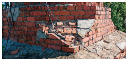
Photo 5. Technical condition of the lower part of the chimney – significant defects in the supporting structure of the chimney above the parapet and elements of wild vegetation are visible
