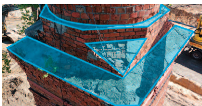
Photo 6. Method of securing the parapet and sloping surfaces at the bottom of the chimney, the blue colour indicates the surfaces to be secured with restoration mortar
