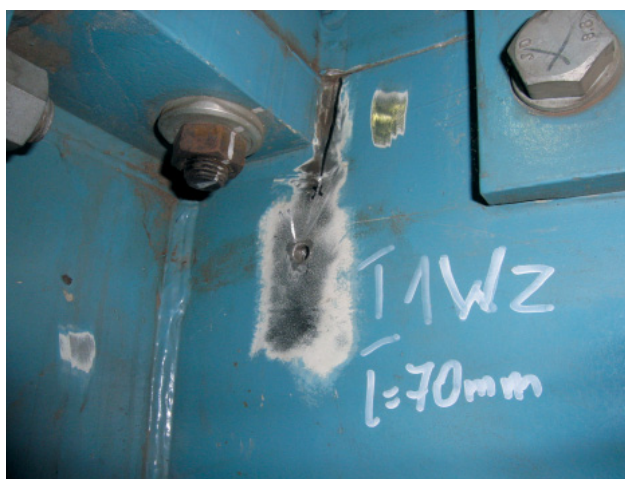
Fig. 2. Crack on the contact point between the shield and the side disc
