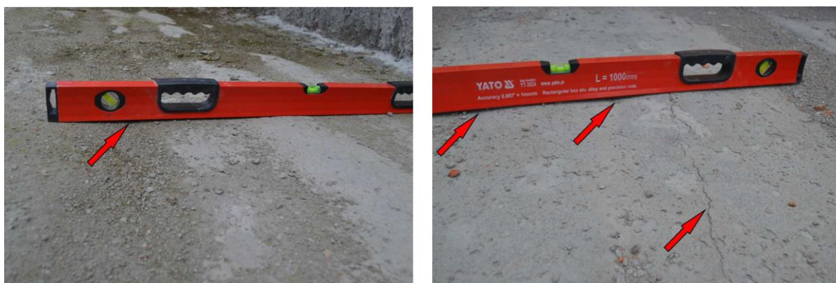
Figure 4. Disadvantages of the process of forming elements, collapse of concrete in the zones of channels and local longitudinal scratches
