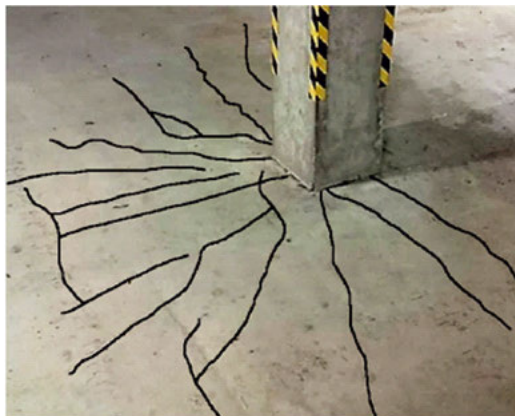
Fig. 13. Crack pattern in the upper surface of the floor slab close to column
