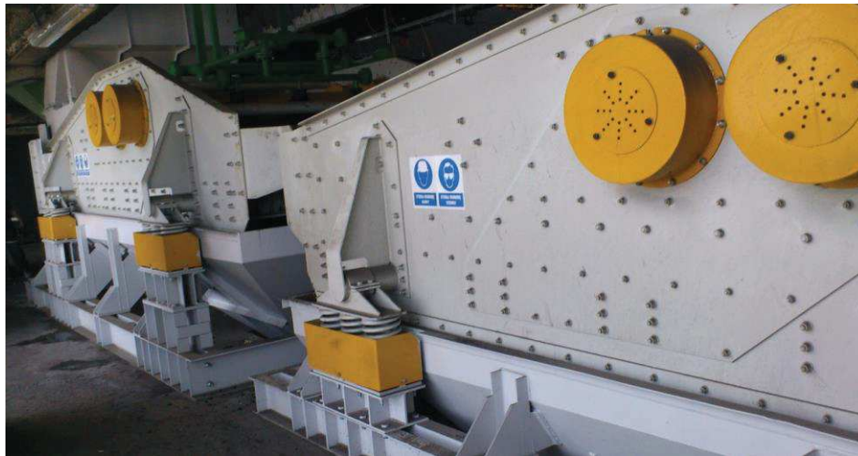
Fig. 11. DISA concentrator coal output, feed to dewatering and sorting sieve
