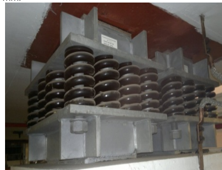
Figure 10. View of vibration isolation package for one of the columns
