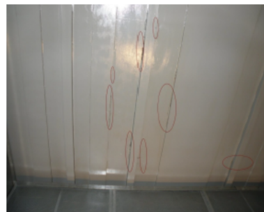
Figure 1. General view of a part of a damaged structure of the considered generator's bottom plate
