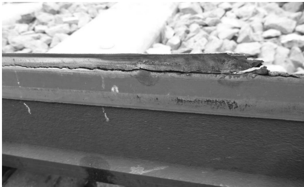
Fig. 4. Crack propagating near spallings of material of the switch rail [photo. M. Czarnecki]
