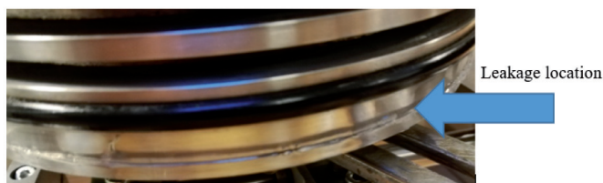
Fig. 5. View of the working fluid leakage
