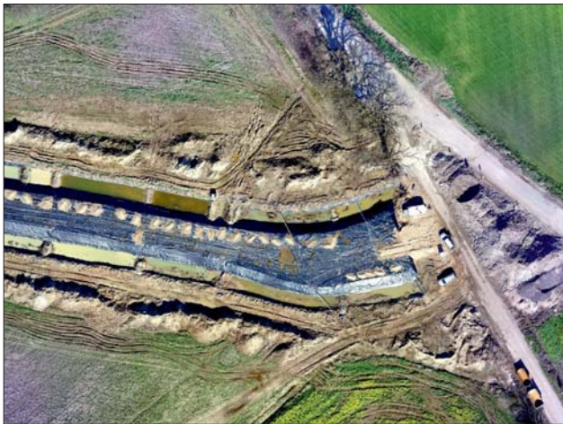
Ryc. 6. Fragment terenu badań w trakcie budowy drogi Fig. 6. Part of the investigation area during road construction
