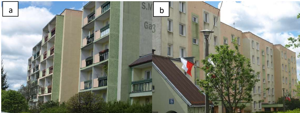
Fig. 1. Facades: a) southern, b) northern of a residential building constructed in the Wk-70 system
