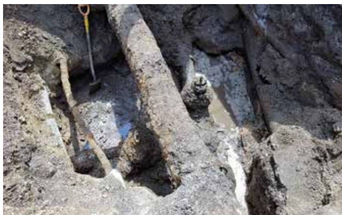
Fot. 6. Gate tee, prepared to be replaced (over and next to the tee, the pipelines of rain sewage and, also, telecommunication cables in protection tubes are visible)
