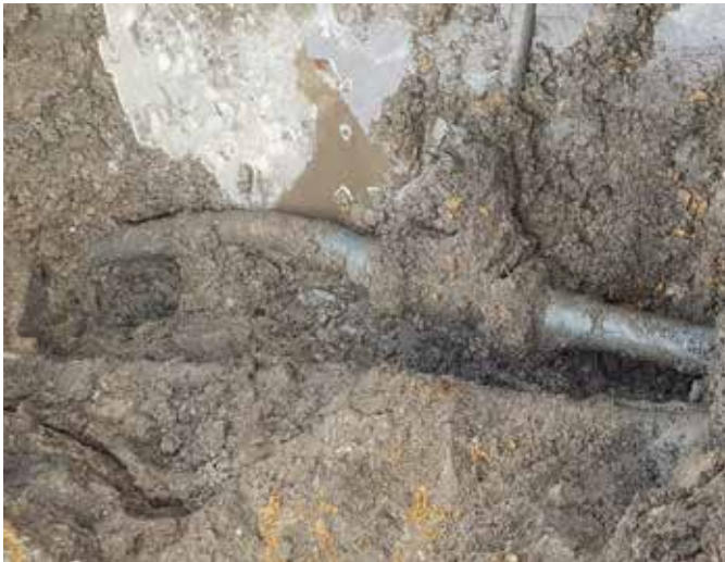
Fot. 4. Rupture in the area of tee joint in the distribution PVC network
