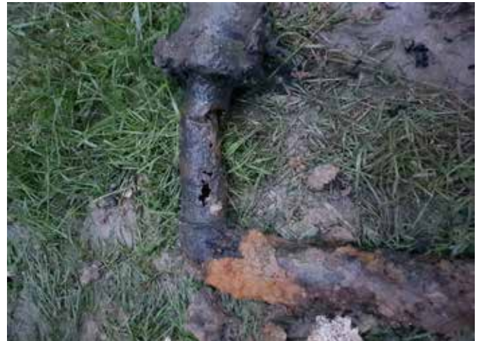
Fot. 1. Point corrosion of water pipeline connection
