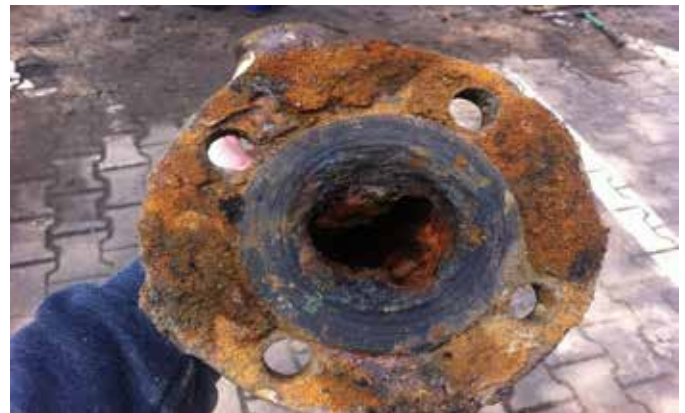
Fot. 2. Image of corrosion inside the steel pipeline
