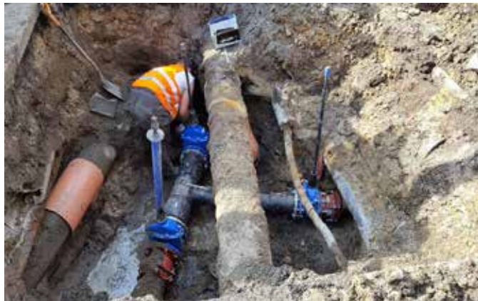
Fot. 8. The replaced gate tee (before recovery of the correct water flow, the worker visible in the photo, is checking the force of tightening the screws)
