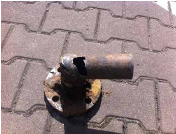
Fot. 3. Image of point corrosion
