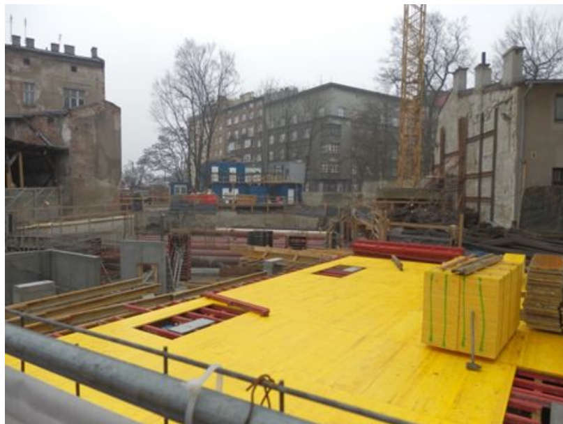
Fig. 3. The building site of the new multi-family building in the vicinity of the Kossakówka manor and park, view from Wygoda Street. Photo by R. Łabuz, 2016.
