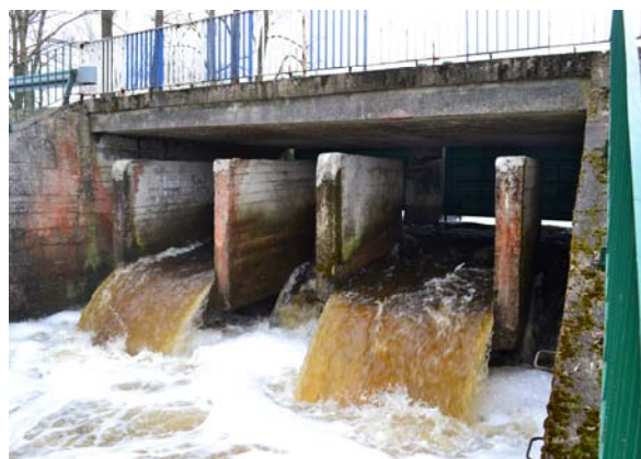
Photo 1. View of the multi-chamber weir in Glinny Stok village (phot. A. Mazur)
