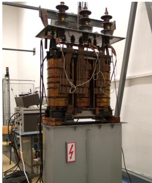
Fig. 1. Experimental transformer BEZ aT0294/22 Yzn1.
