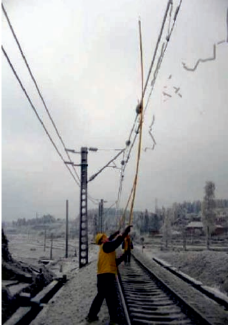
Fig. 2. Mechanical de-icing of the catenary with an insulated rod [2]
