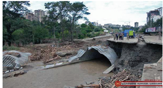
Fig. 4. Newly built tunnel broken by water flow (photography by Robert Diakonidze)
