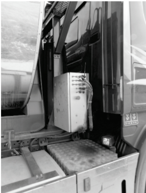
Fig. 9. a) control panel b) RECO-DRIVE system (from the authors' collection).
