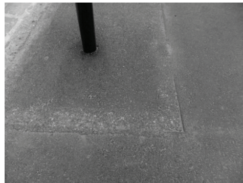
Fig. 5. Examples of pavement defects - raveling (from the authors' collection).
