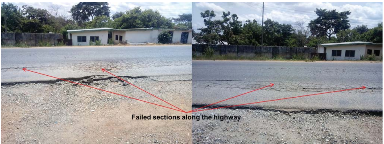
Fig. 2. Parts of failed sections along the highway in the study area.
