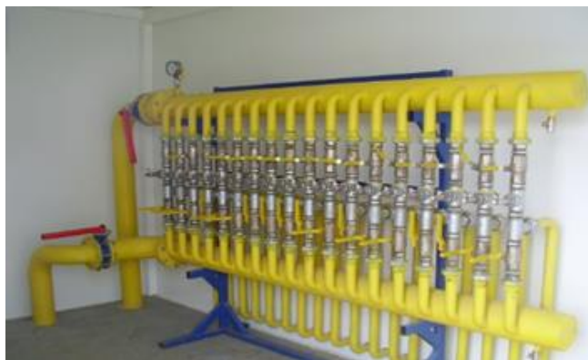
Fig. 3. Connection of gas wells to main pipelines (13)
