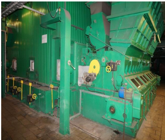
Fig. 1. The boiler type WR-25
