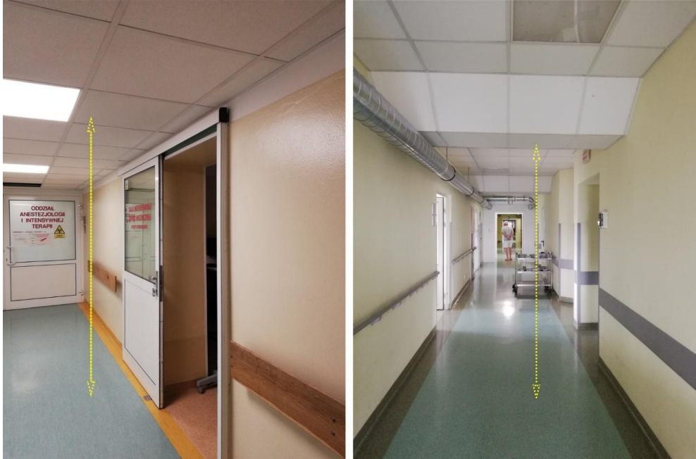
Fig. 7. Picture on the left – maximum lowering of the false ceiling to hide the installation ducts above the false ceiling – the result is a room that is too low according to the regulations, with a disturbed scale (quite claustrophobic). Photo right – unusual shaping of false ceilings in place of pull-ups, ventilation ducts routed under the false ceiling, in a conspicuous location, significantly detracting from the aesthetics of the ward, Puławy, developed by the authors, 2022
