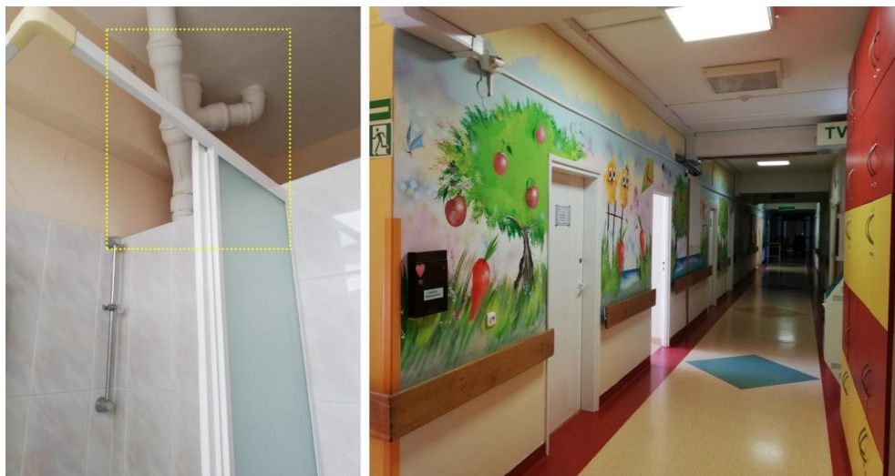
Fig. 8. Photo left – no replacement and no changes to plumbing. Photo right – arrangement of the children's ward, made with low-quality materials, without consideration of colour selection, resulting in a chaotic, aggressive and incoherent interior, Puławy, prepared by the authors, 2022
