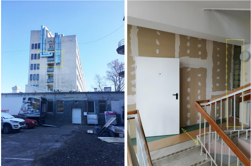
Fig. 4. Conflicts and problems associated with the partial view of the modernisation. Photo left - mechanical ventilation ducts routed through loggia, across elevation to the roof. Photo right - stairwell partition wall introduced as a result of Covid zoning, limiting the extent of the stair landing and terminating at the location of the glazed existing wall, Puławy, taken by the authors, 2022.
