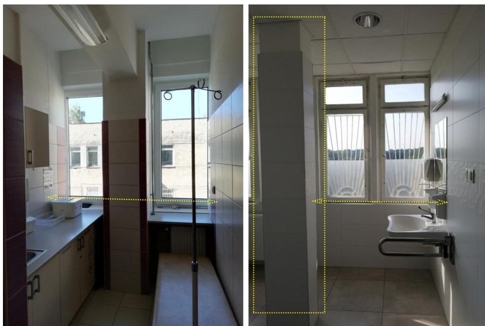
Fig. 6. Photo left - treatment room width too narrow, due to the location of structural walls and the grid of prefabricated columns, new windows not adapted to existing condition (collision with walls). Photo right - disabled toilet, in the middle of which is an enclosed sewer riser from the upper floor, Puławy, prepared by the authors, 2022
