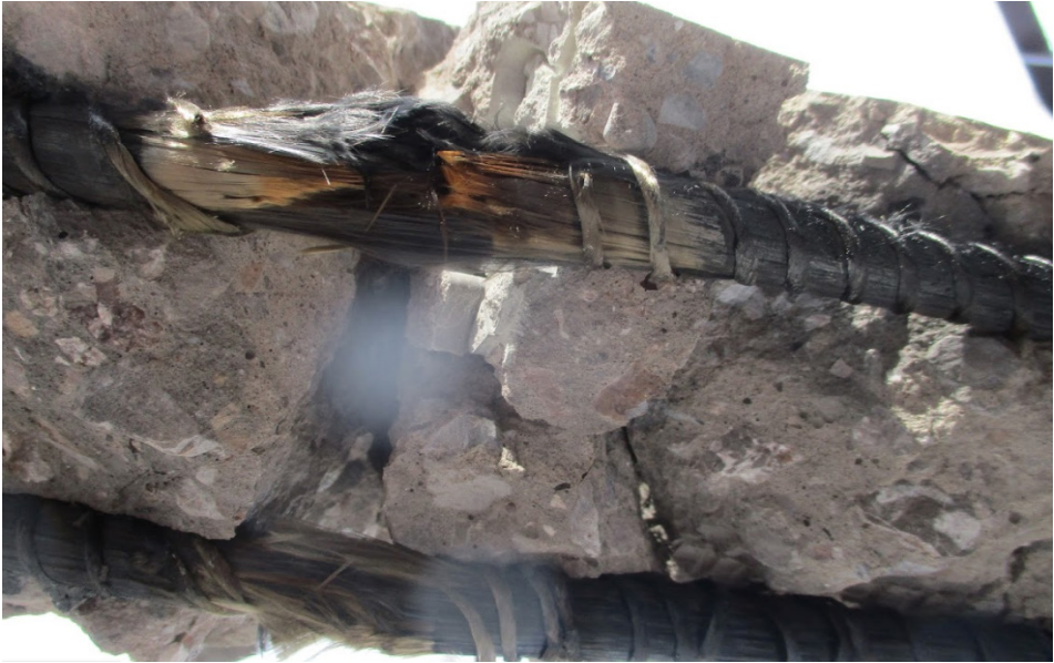
Fig. 4. Uncovered HFRP bars (by removing the clear cover after testing). Source: own study
