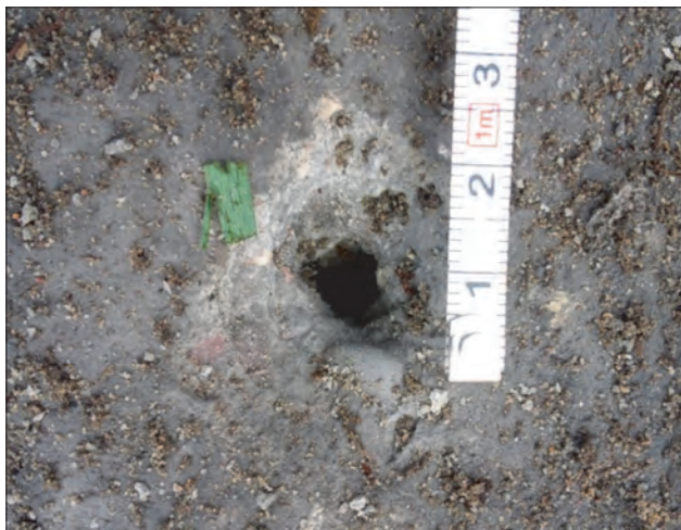
Fig. 11. Photograph of inlet in a concrete slab after firing with a shaped charge containing a semi-spherical liner made of an iron-based alloy
