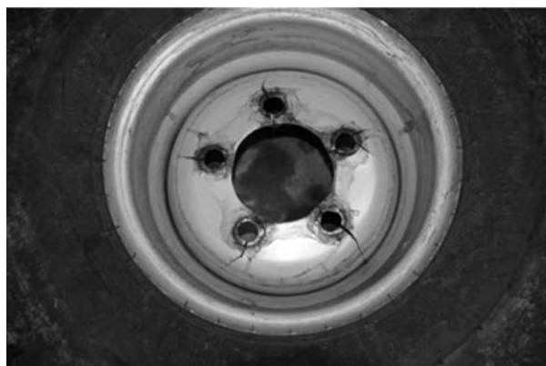
Fig. 1. A view of a wheel rim with cracks formed on the mounting holes in the wheel disc
