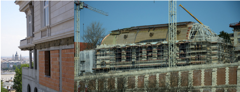
Fig.9 Buildings under reconstruction on the Castle hill of Budapest: Lónyay villa (around 2000) and the Riding School (2018); Photo: Ádám Arnóth
