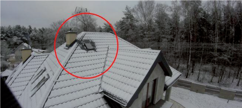
Figure 5. Picture of roof window, shoot from the west. Visible heat losses around the window [zdj. T. Sasin, 2014]
