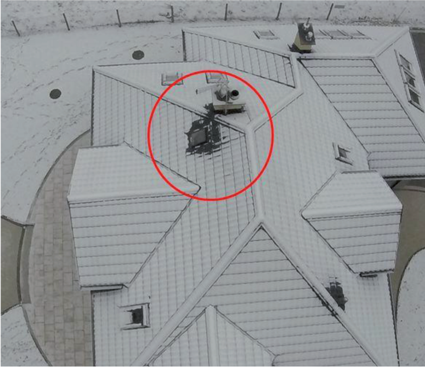
Figure 13. Picture of the whole building from the south side. Visible heat losses around roof window, placed on the west side [zdj. T. Sasin, 2014]
