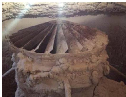
Figure 1. Scaling on the distributor in the desulfurization tower
