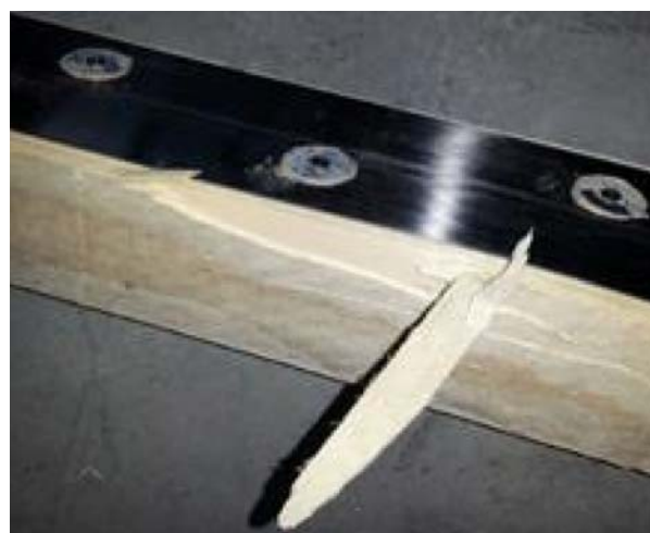
Fig. 14. Detail of the typical failure mode of reinforced beams
