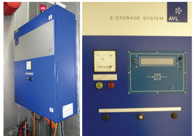
Fig. 5. The equipment used during testing: AVL e-storage (power battery unit)
