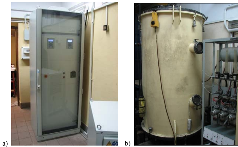
Fig. 7. Modernisation of a production line in “Motor” company (a – ion nitriding module, b – technological stand)
