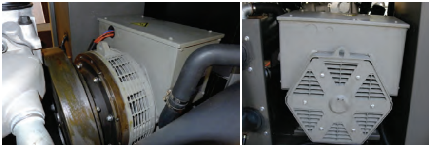
Fig. 5. CHP unit current generator (view from and towards the engine)
