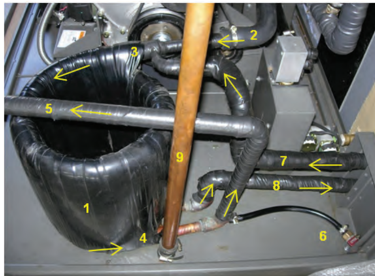
Fig. 7. Operating heat exchanger for heated water external system 1 – heat exchanger, 2 – coolant pipe from second heater on the exhaust pipe, 3 and 4 – start and end of parallel pipe system of engine cooling system (heat source) and external system (heat receiver), 5 – coolant pipe to engine radiator, 6 – valve for emptying engine cooling system, 7 – pipe with water to heat from external system, 8 – pipe with heated water to external system, 9 – overflow pipe carrying off water from the upper unit chamber, arrows – coolant and heated water circulation
