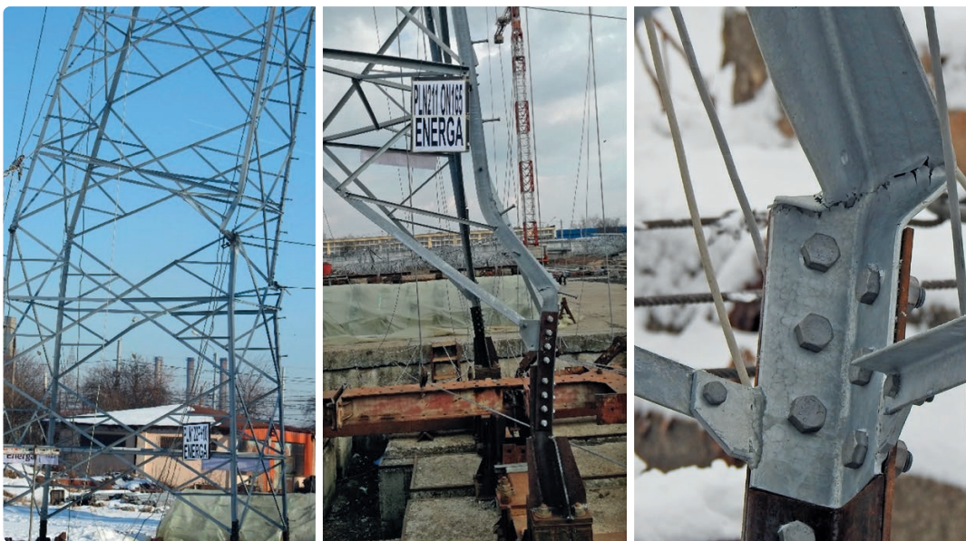
Photo 2. Damaged supports: PLN122 P (left), PLN 122ON165 (centre), and PLN211 P (right)
