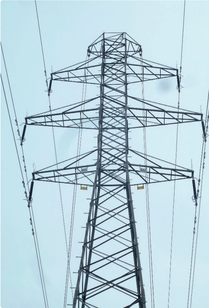
Photo 3. PLN211 P tower of the 110 kV line to Daszyna substation
