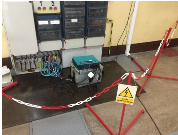
Fig. 24. Place and method of connecting the power quality analyzer Memobox 800
