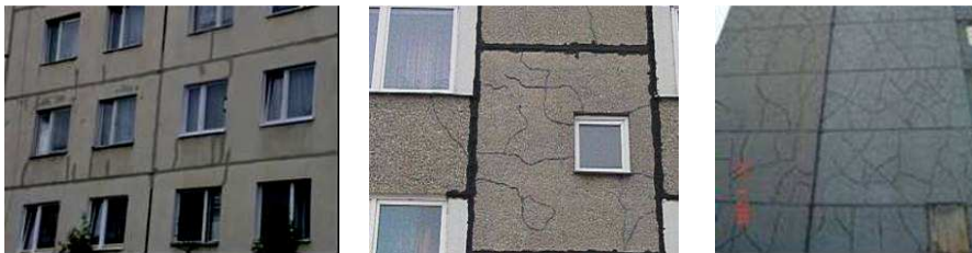
Fig. 9. Examples of characteristic crack patterns in texture layer
