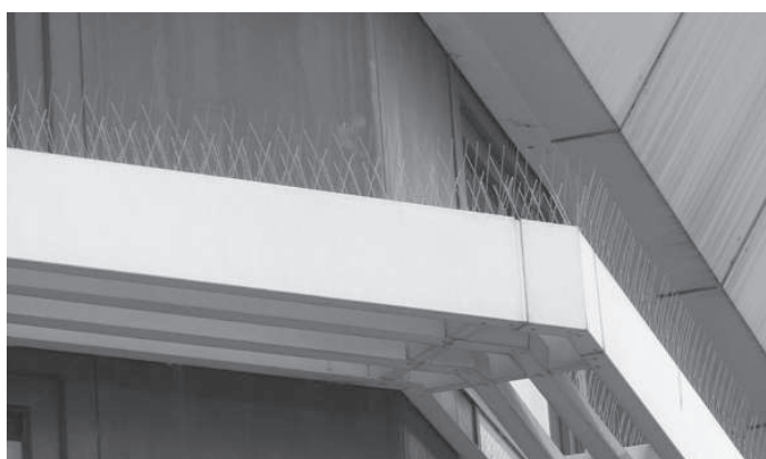
Photo 1. Protecting nets on cornices of the SGGW building
