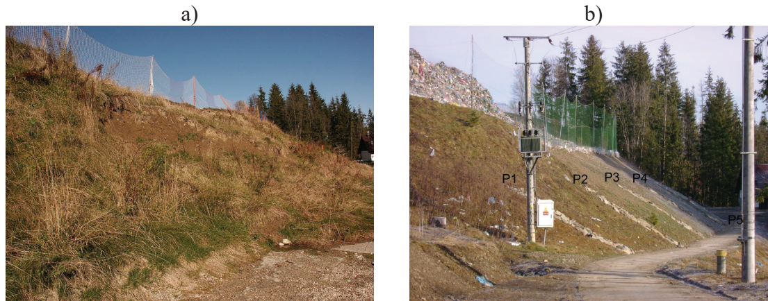
Figure 2: Landfill retaining embankment: a) damaged, 2004, and b) after repairs with counterforts P1–P5, 2005.
