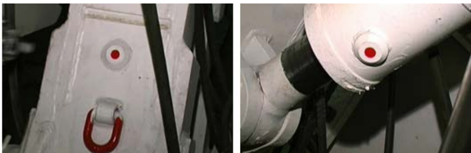
Fig. 2. Examples of installation of TRID-01 transponders on the support components [3, 4]
