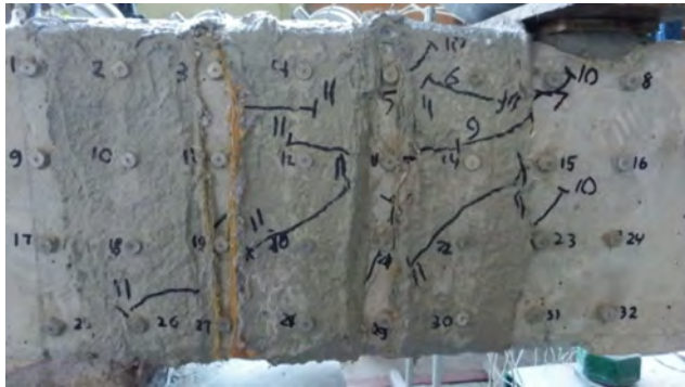
Fig. 8. Distribution of cracks on the surface of the strengthening
