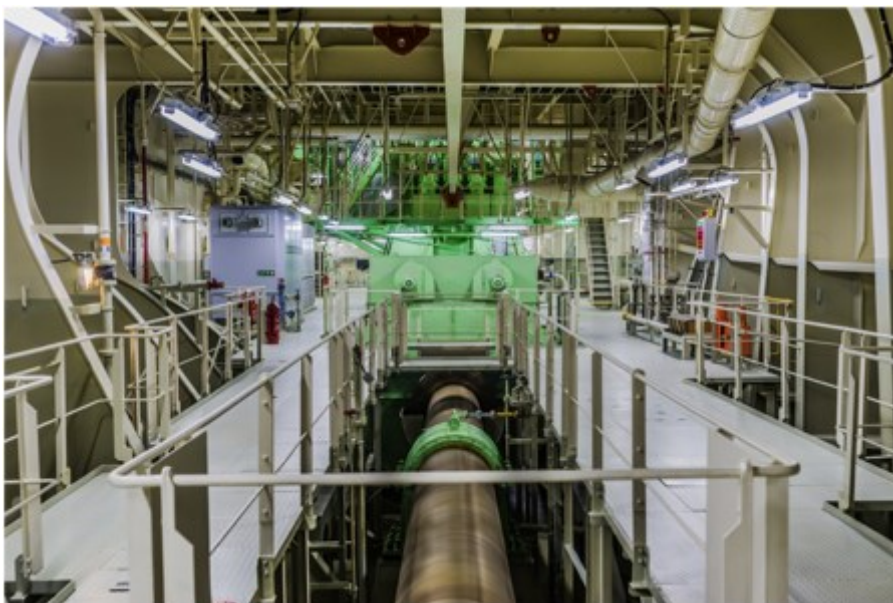
Fig. 2. Mayview Engine Room.
