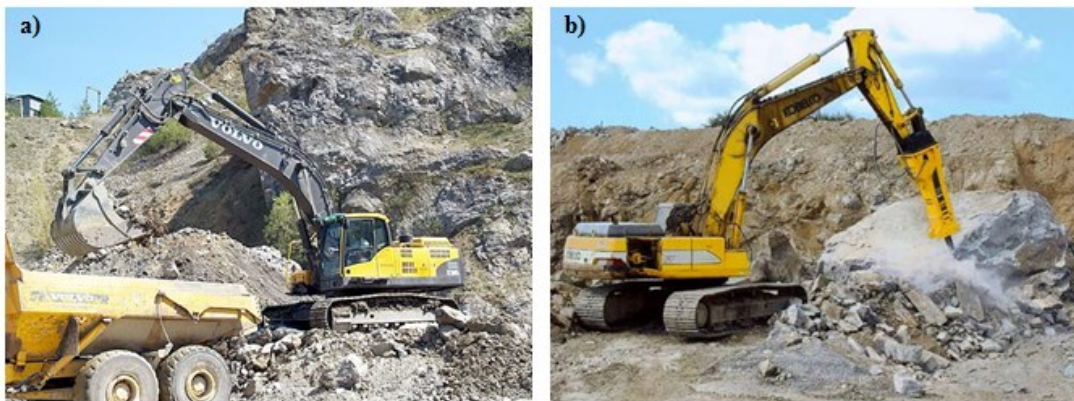
Fig. 1 Single-bucket excavators in the mines of rock raw materials carrying out: a) loading, b) shredding oversized lumps
