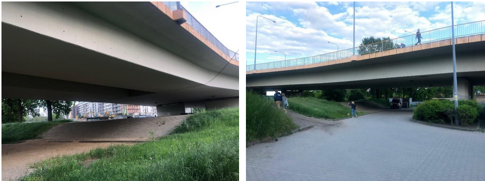
Fig 10. Photos of the examined area. Milenijny Bridge (left-bank flyover) – crossing over the Odra River with access roads as part of the city-centre bypass, the section from Legnicka Street to Osobowicka Street, Wrocław – span № 6, between 6 th and 7 th axis – measurement axis #1. Source: author's Elżbieta Komarzyńska-Świeściak own photo archive
