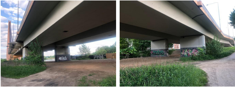
Fig 9. Photos of the examined area. Milenijny Bridge (left-bank flyover) – crossing over the Odra River with access roads as part of the city-centre bypass, the section from Legnicka Street to Osobowicka Street, Wrocław – span № 7, between 7 th and 8 th axis – measurement axis #2. Source: author's Elżbieta Komarzyńska-Świeściak own photo archive
