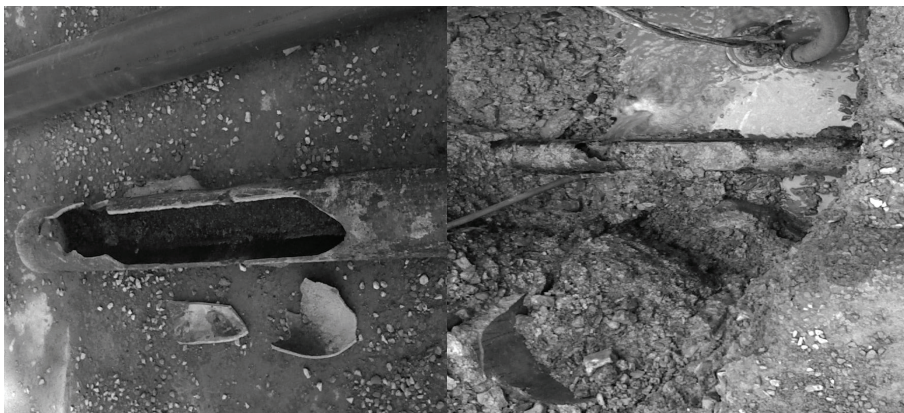
Fig. 1. The example of influence of soil properties to corrosion of water pipe (own study)
