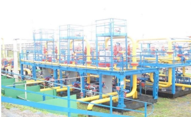
Fig. 2. Piping of the main lines and measuring lines at CGTU-2 of the Yuliivske OGCF
