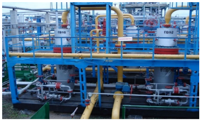
Fig. 3. Separators piping at the main line at CGTU-2 of the Yuliivske OGCF
