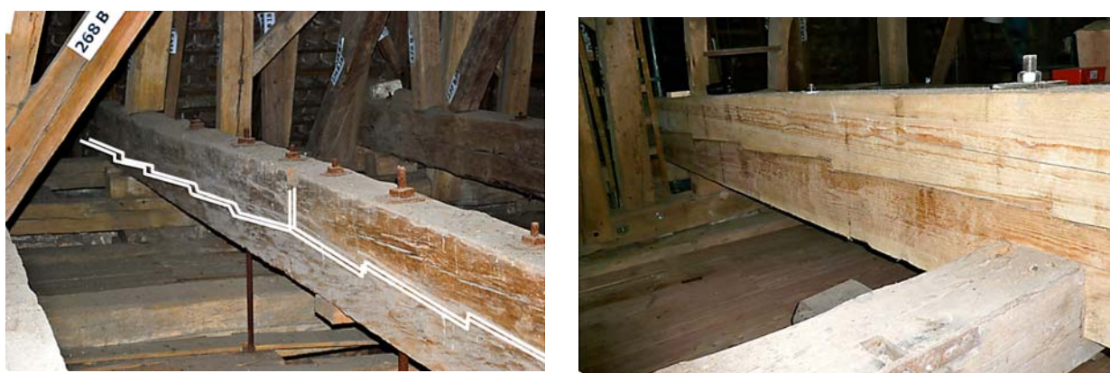
Fig. 3. Left: 270 years old teathed beams as upstand beams; right: true to original reproduced teathed beam (wood species: pine)
