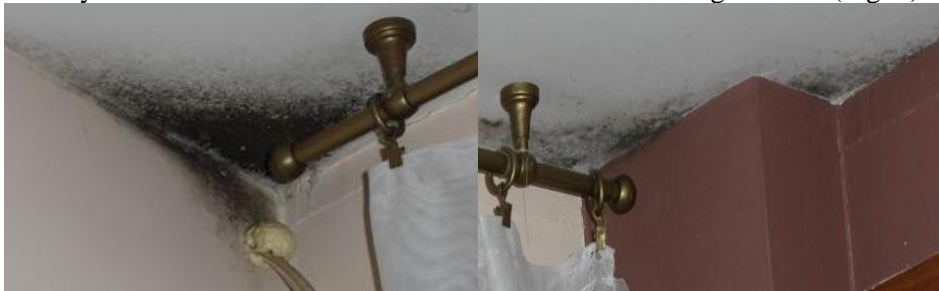
Fig. 5. Mold-covered upper wall corner below the balcony and ceiling comprising an extension of the balcony
