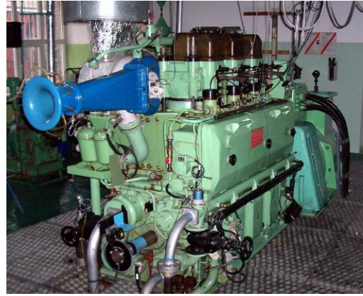
Fig. 1. Test bed with Sulzer 3AL 25/30
